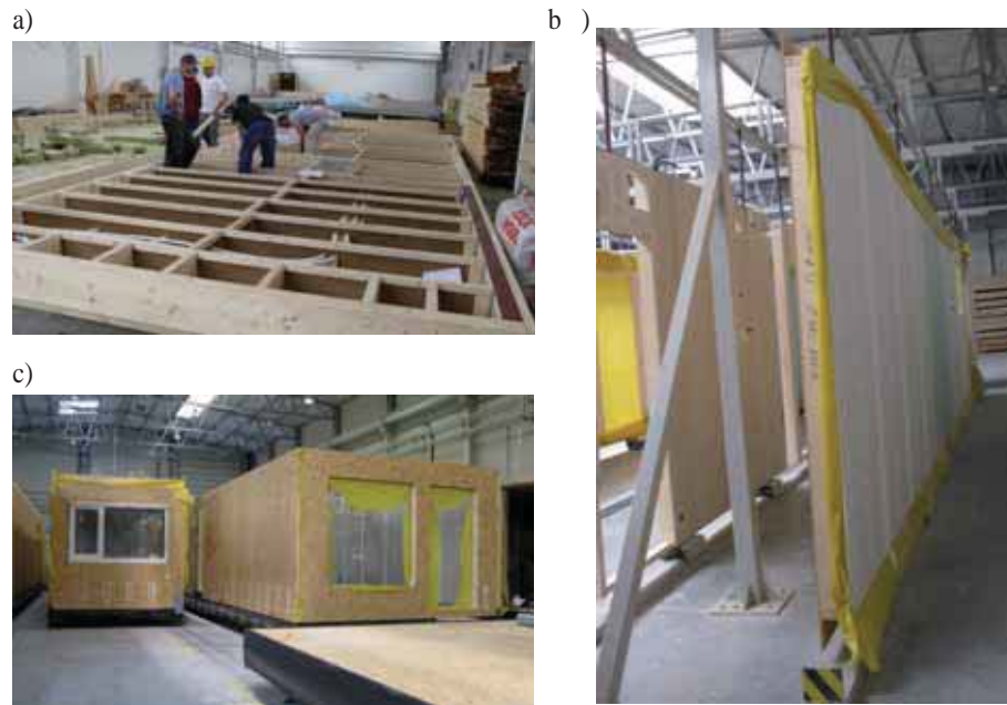
Fig. 8. Stages of module assembling: a) sub-assembling of floor elements, production of wall panels, c) assembling of module structure (UNIBEP)
