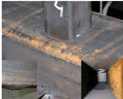
Fig. 5. Joint WT2L4 after test (detail of face wall failure in right corner).
